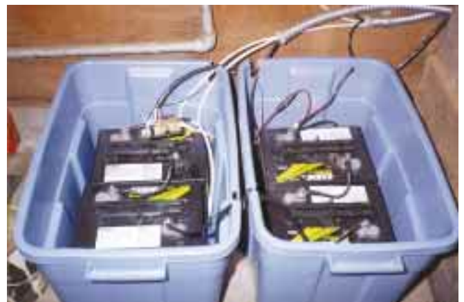
Below: Exide T-105s in spill-proof tubs.
