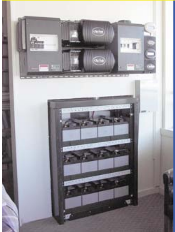
This state-of-the-art installation provides clean, renewable energy and serves as a fantastic demonstration system for the public to see firsthand.
