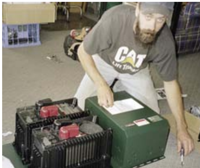
Installer Ben Scurfield assembles the OutBack PS2 power panel. The second inverter case is for display only.
